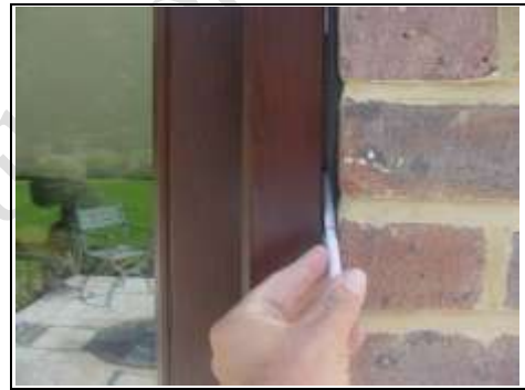
Mastic not applied
