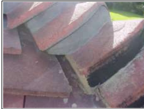
Poor ridge tiles detailing
