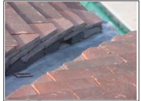
Valley gutter starting to deteriorate
