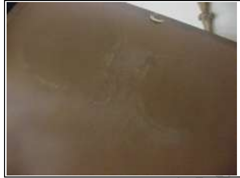
Mould appearing on the back of the pictures in the lounge
