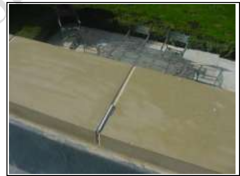
No DPC to coping stone a way around this would be capping the coping stone or removing it and adding a DPC and replacing it with a suitable coping stone.
