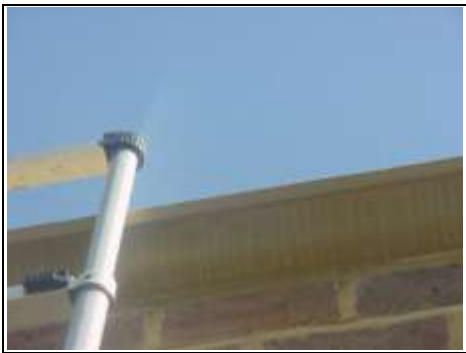
No drip detail to the front of the coping stone allowing water ingress into the property
