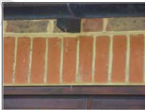
Water missing the gutters and coming down the wall
