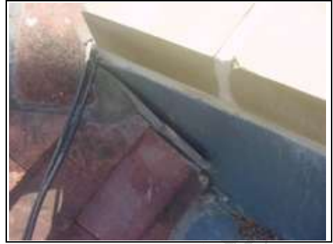
Poor lead gutter detail
