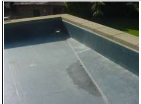
No fall on roof towards the hopper heads and downpipes
