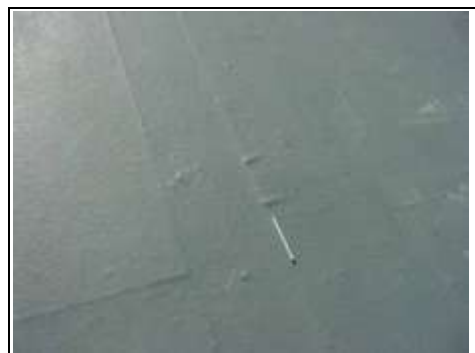
Blistering in the flat roof
