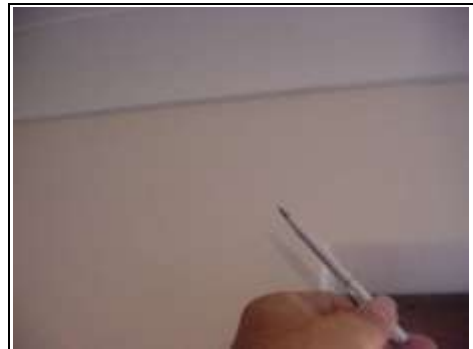
Cracks visible in the adjacent bedroom
