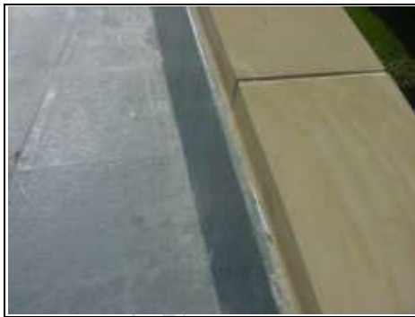
No drip detail to the coping stones
