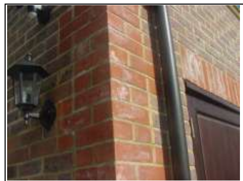
Efflorescent on the bricks
