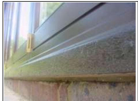
Wood under the window has not been stained
